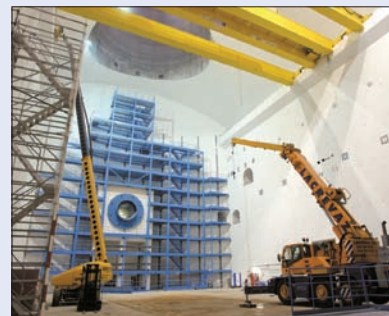
The ATLAS cavern was handed over to CERN by the civil engineering contractors in a ceremony on 4 June 2003. This 12 storey access structure was one of the first items installed.
