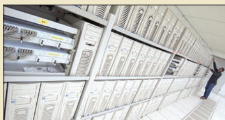
The machine room of CERN's computer centre.
