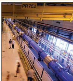
A complete LHC cell of six dipoles, straight sections, a prototype cryogenic distribution line and an electrical feedbox began tests in the full String 2 June 2002.
