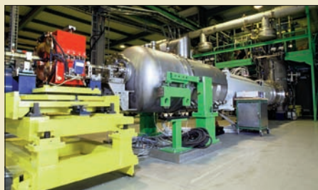
A short straight section, containing a prototype LHC main quadrupole, on its testbench at CERN.
