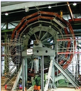
The first ring for the barrel yoke of the CMS superconducting magnet under assembly in 1999 by the manufacturer Deggendorfer Werft und Eisenbau GmbH (DWE) in Germany.
