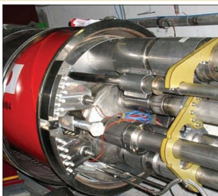
On 13 July 2007, an inner triplet assembly of quadrupole magnets passed its pressure test in the tunnel after strengthening modifications.
