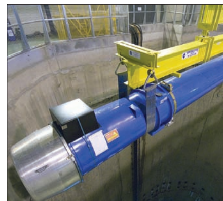
The final superconducting magnet system, 15 m long and weighing 34 tonnes, made its descent into the accelerator tunnel on 26 April 2007.
